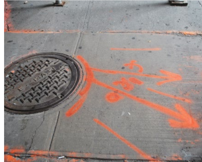
Level 3 Communications manhole and cable markings, lower Manhattan, 2014. Photograph by Ingrid Burrington.
