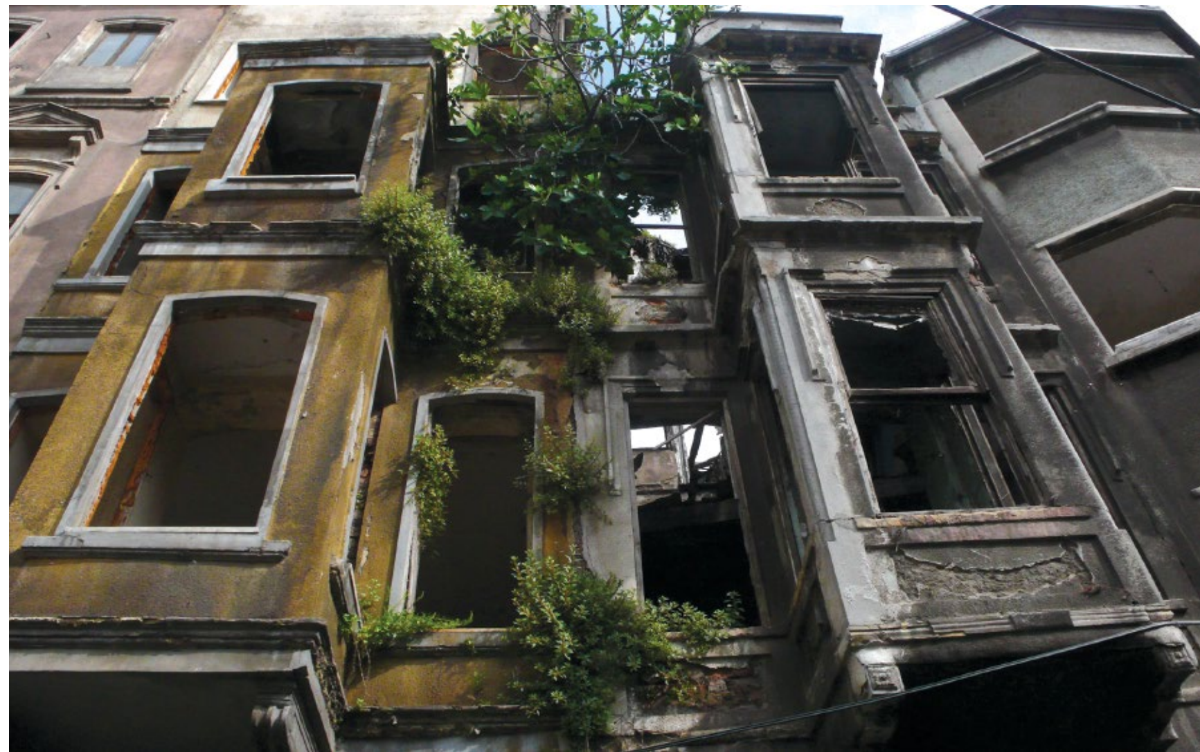
Gregory Buchakjian, photograph of Istanbul's Tarlabasi neighborhood that was due to be demolished. May 6, 2013, a few weeks before the Gezi Park demonstrations started. Courtesy of the artist.
